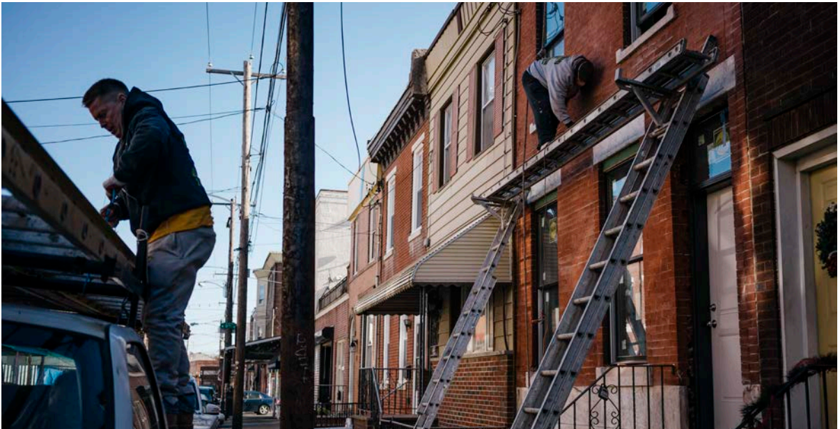
Masonry workers restore a home's façade in South Philadelphia. A new Pew initiative will focus on fresh approaches to helping people find affordable housing and mortgages. Lexey Swall for The Pew Charitable Trusts
